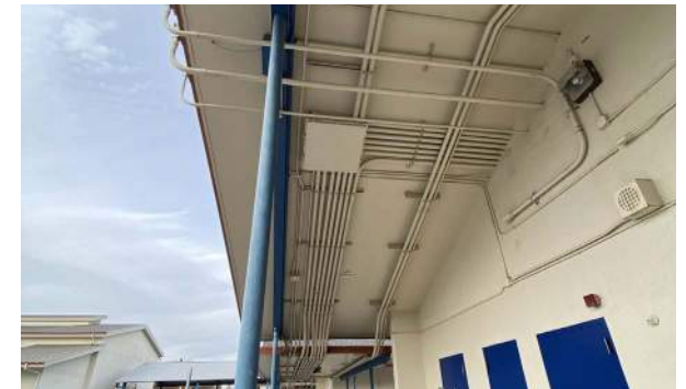
Utilities at Covered Walkway
